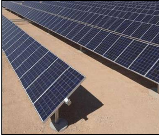
Figure 2 – strings of single-axis solar trackers
